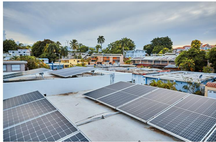
Sunnova solar installations in Puerto Rico.
